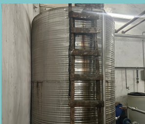
A Recovery Steam Storage Tank
