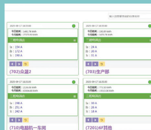
A Real Time Monitoring System
