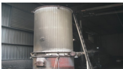
Boiler with organic heat carrying agent
