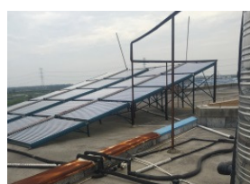
Solar water heater
