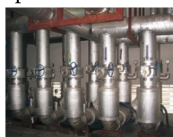
Ice-cooling storage system's pipes
