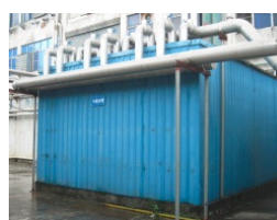
Ice storage tank
