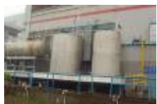
Collection of water condensate
