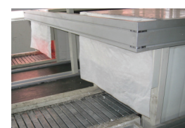
Thermal insulators at heaters
