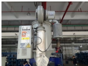
Heat Recovery for dryer (Before Improvement)
