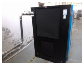
Variable speed screw air compressor with permanent magnet motor
