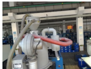
Heat Recovery for dryer (After Improvement) – Red ducts
