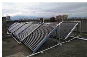
Solar heater panels
