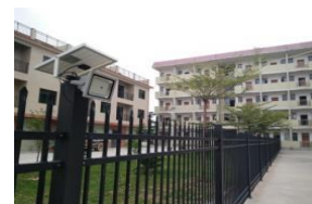
Solar street light
