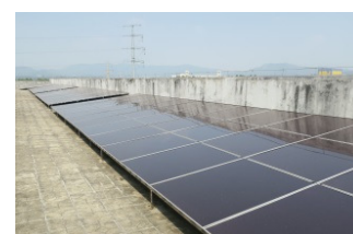
Solar PV panels
