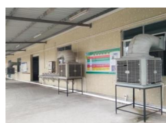
Water-curtain HVAC system
