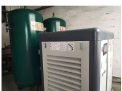
VFD air compressor
