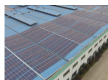
Solar PV panels
