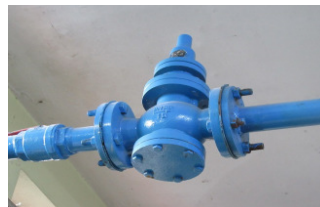
Pressure control device in compressed air system
