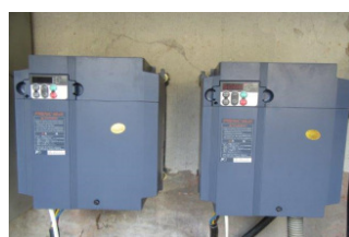
Variable frequency drives in water pumps
