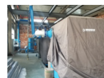
VFD air compressor
