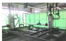
Chamber for water condensate
