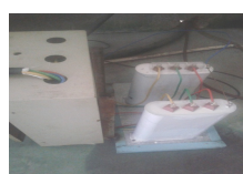
Air compressor - compensated capacitor
