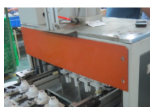
Aging line - baffles
