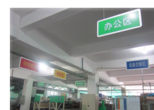
Store room - zone control
